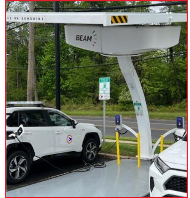
Electric vehicle charging station
