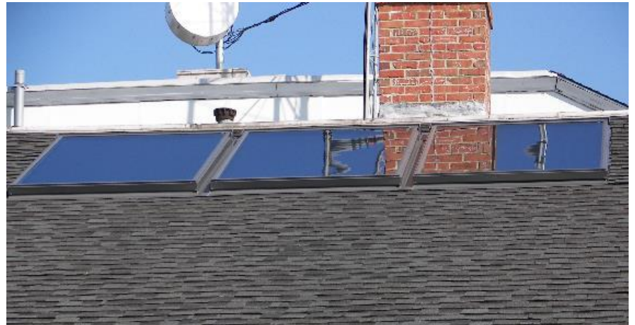
Manchester, NJ solar thermal installation
